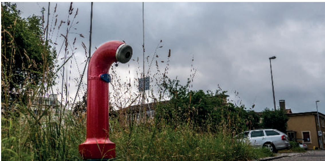
Hydrant Anna Heer-Strasse
